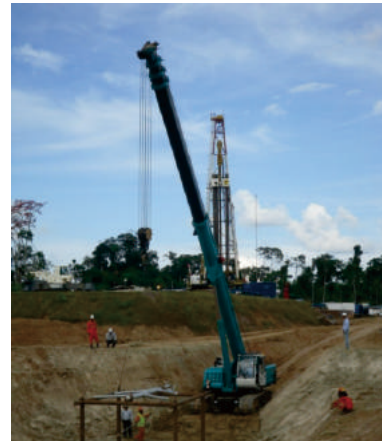
SWTC35在秘鲁施工工地狭小地带作业 SWTC35 Working In Narrow Area In Peru
