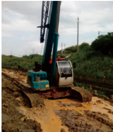
SWTC25在广西南宁沼泽地作业 SWTC25 Construction In Nanning Marshland, Guangxi
